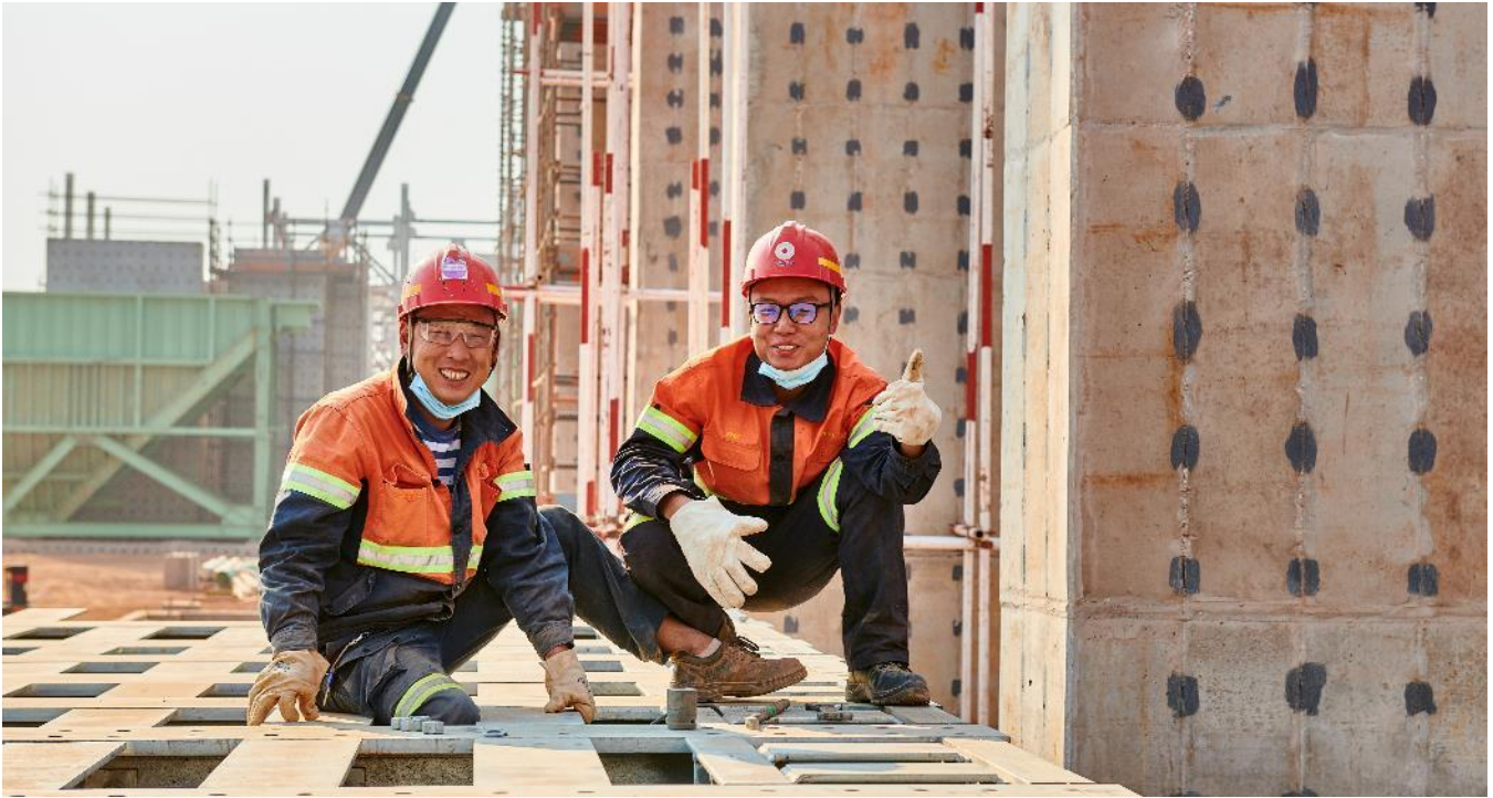
Chen Hong Tao (left) and Wang Pengfei installing the Phase 2 flotation base plates.
