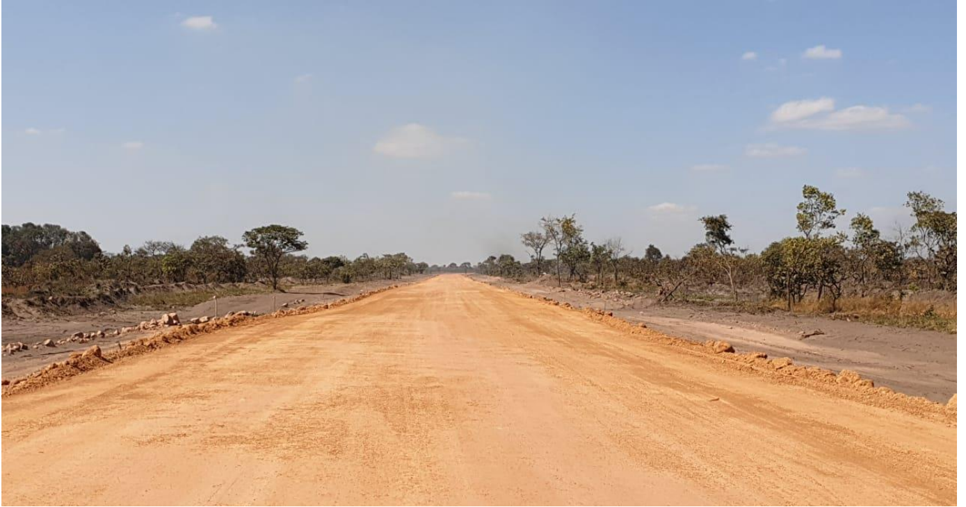
Figures 3 and 4: Ongoing construction work on the new 11-metre wide highway from the Kamoja-Kakula Project to Kolwezi airport, which is designed for speeds up to 80 kilometres per hour.
