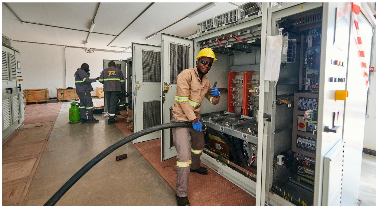
Electrician Tresor Nawej Tshimwish installing an electrical cable at the Phase 2 high-pressure-grinding-rolls (HPGR) substation. More than 83% of the Phase 2 electrical cable has been installed.
