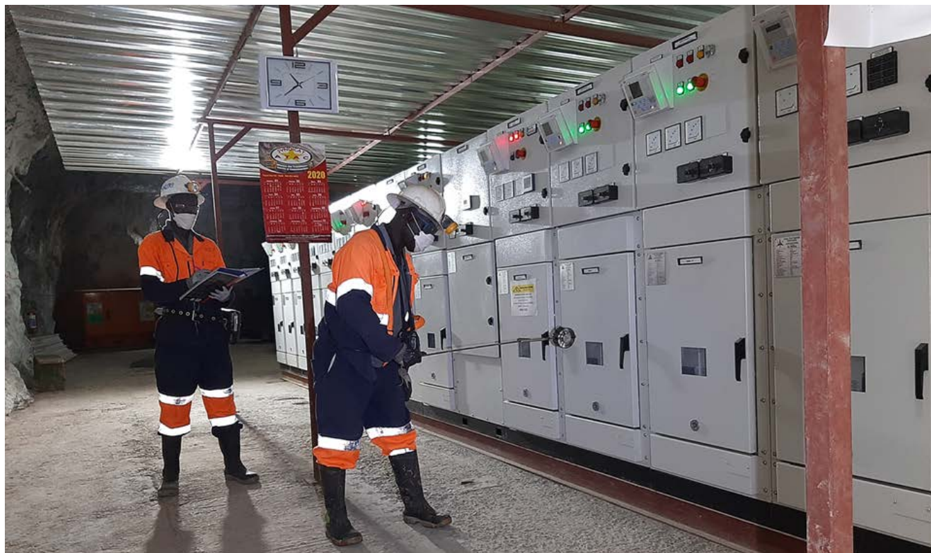
Samuel Ndembo (left) and Mbiya Africa (right) taking air flow measurements at Kipushi's 850-metre-level electrical substation.
