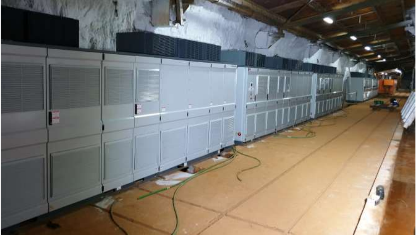
New electrical panels installed underground at Kipushi.
