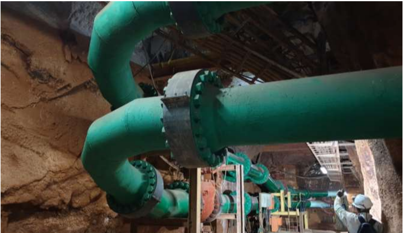
High-volume water pipes to keep Kipushi's underground workings dry.
