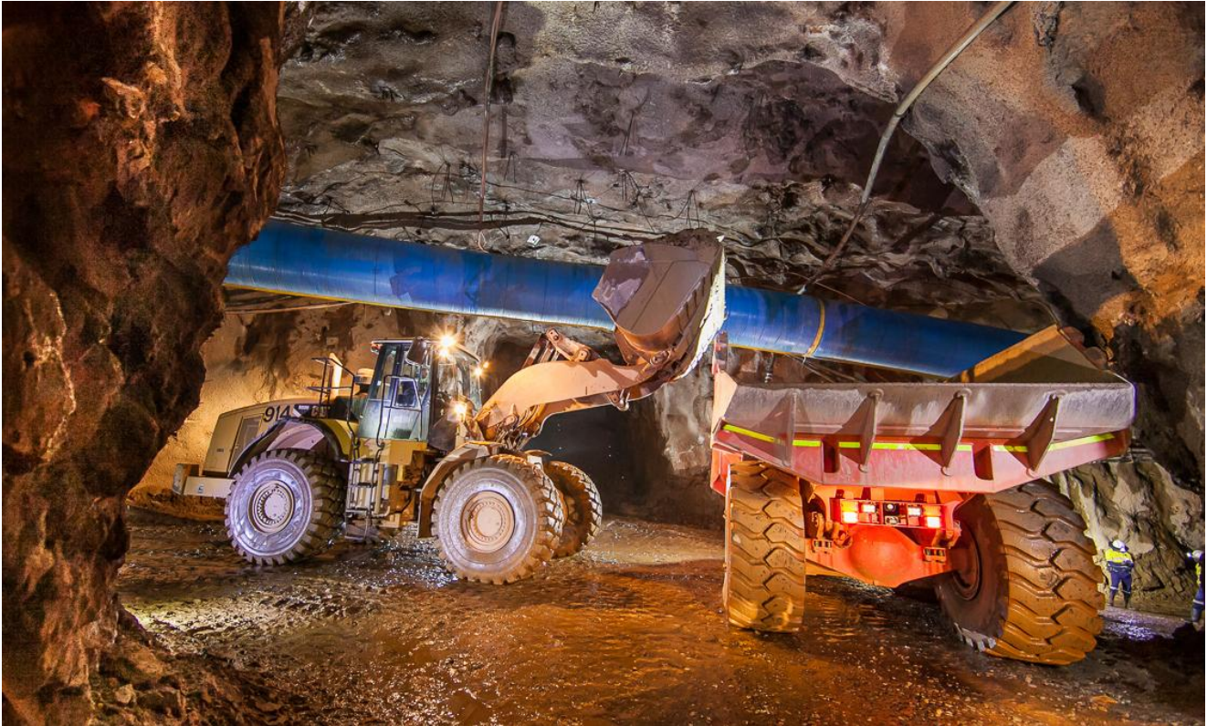
Figure 8. Ongoing construction of access declines for the Kamoia-Kakula Copper Project's high-grade Kansoko Mine.
