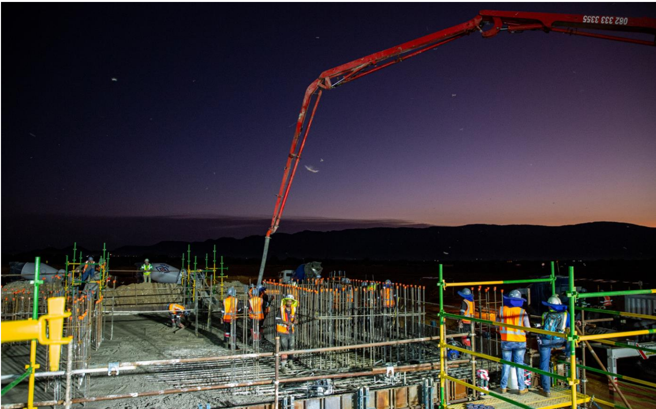
Construction of the foundations of Platreef's Phase 1 concentrator plant is progressing well.
