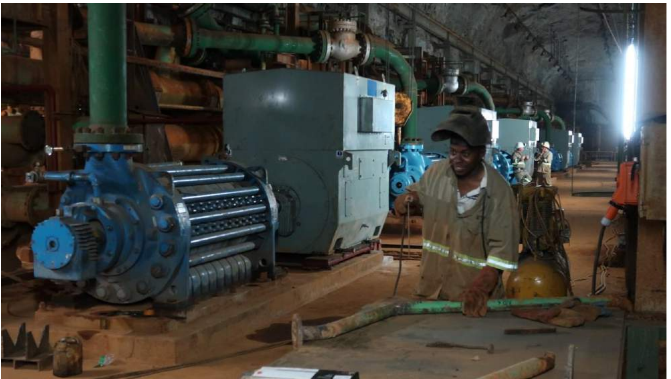
Kipushi's main pumping station at the 1,200-metre level.
