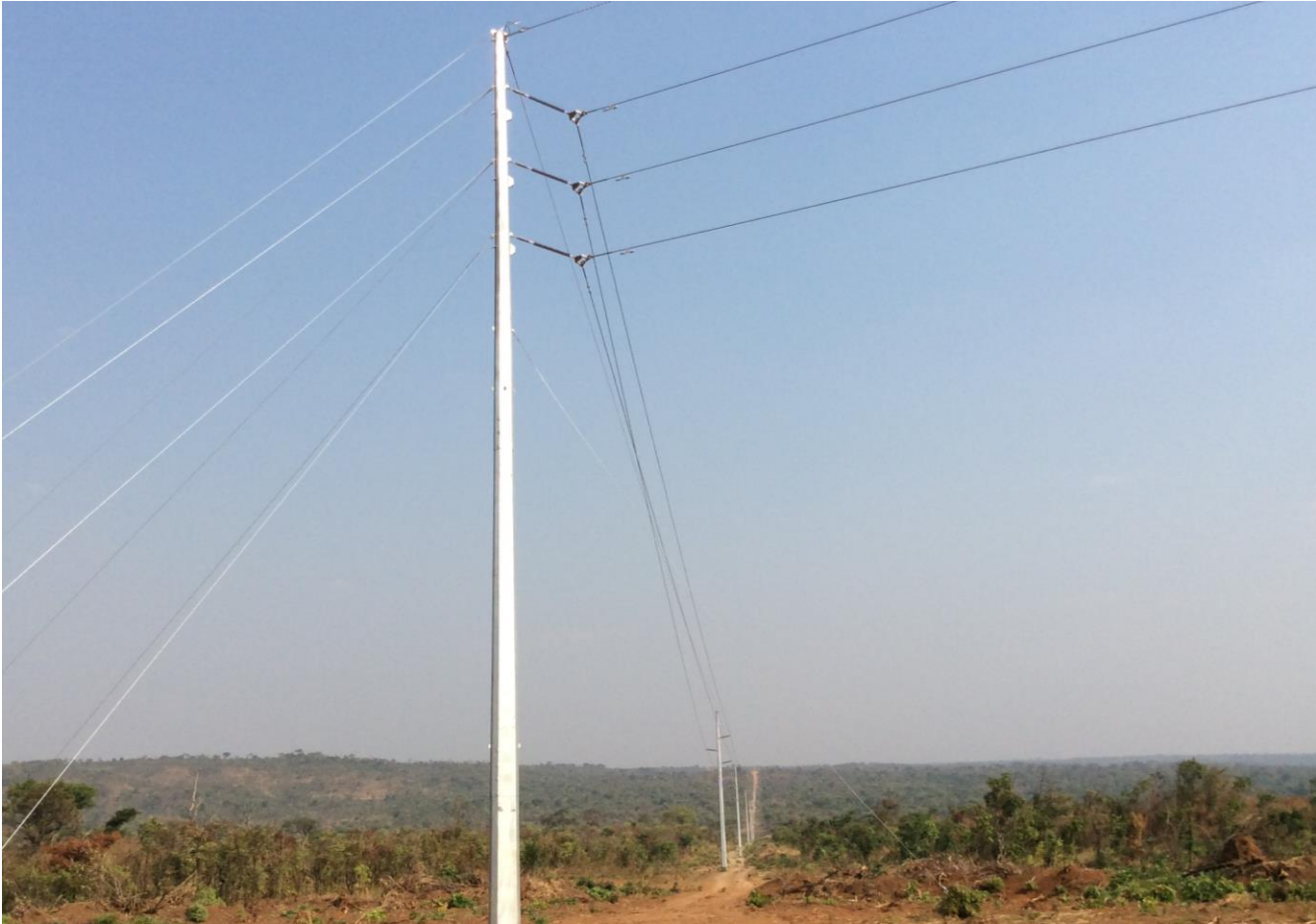
Photo 7. 120-kV power line connecting Kamoia to the national electrical grid.
