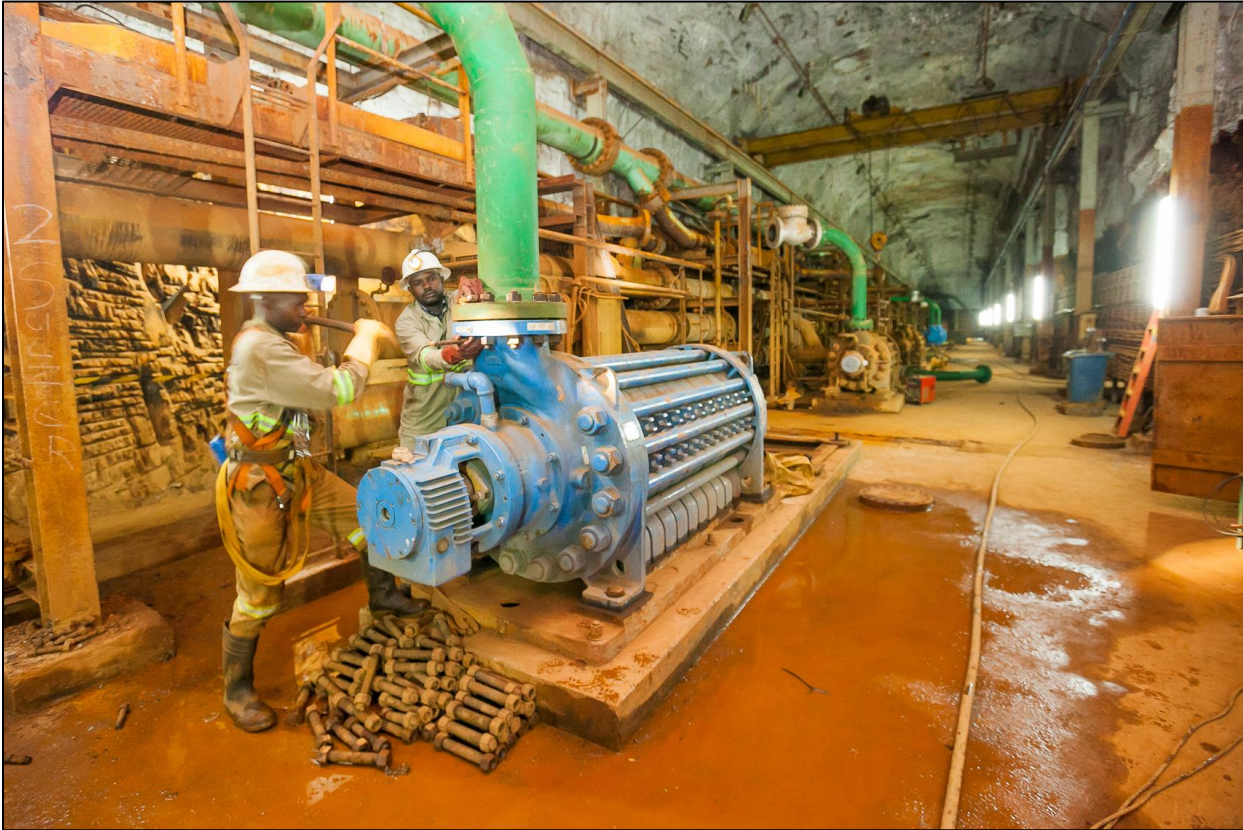
Figure 2. Main pump station in Shaft 5 at 1,200-metre-level with installation of Grifo centrifugal pump.
