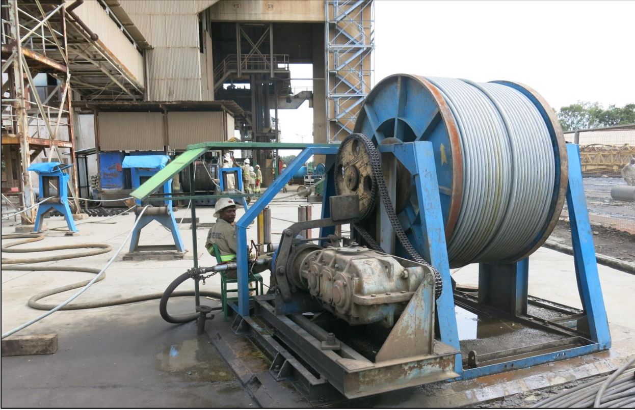
Replacing wire rope on Shaft 5 personnel cage using the friction winder.
