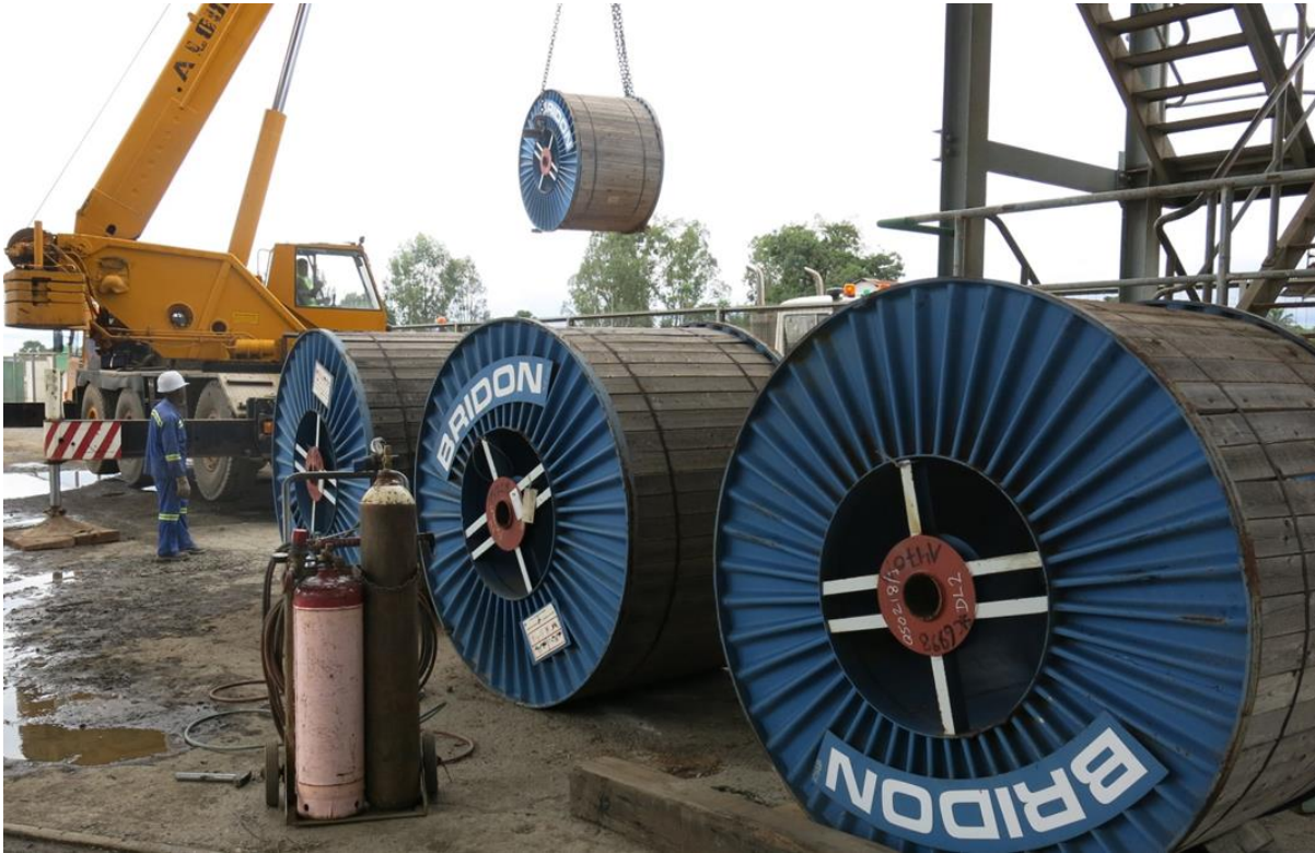
Figure 12: Delivering the new cable for the Shaft 5 man winder.
