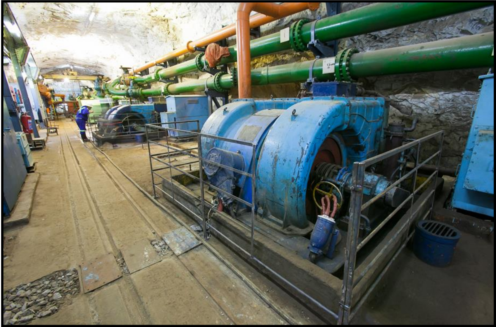
Figure 3: Pumping station at the 850-metre Operations level.
