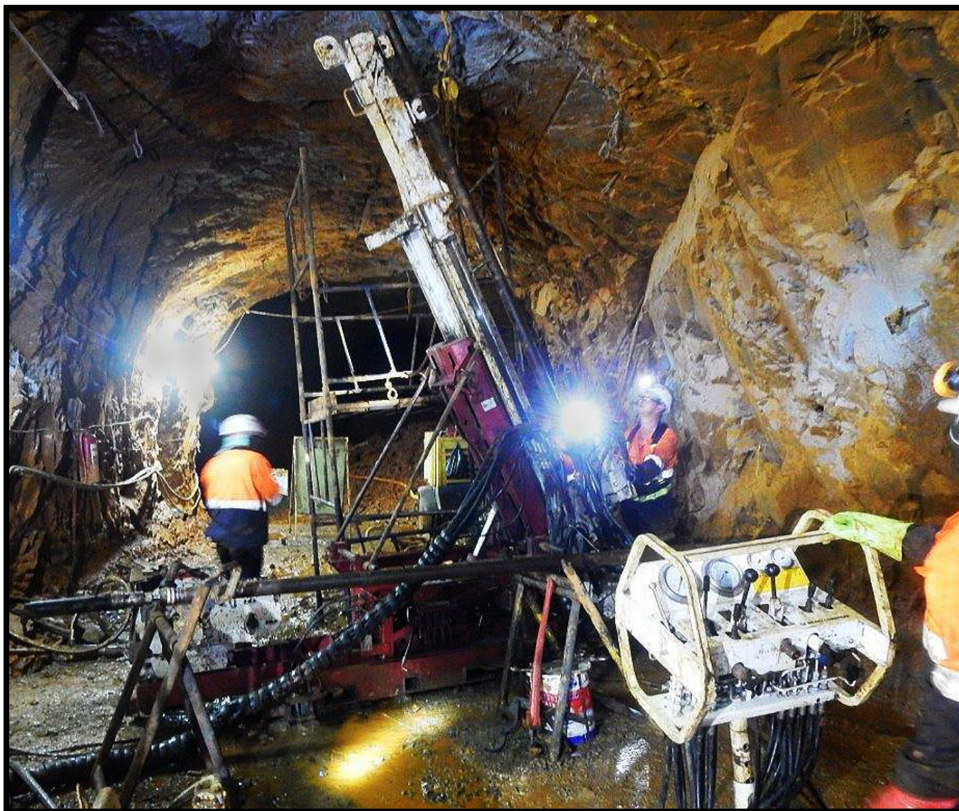
Figure 2: Start of the Kipushi drilling program on March 1 and first drill core out of the ground.
