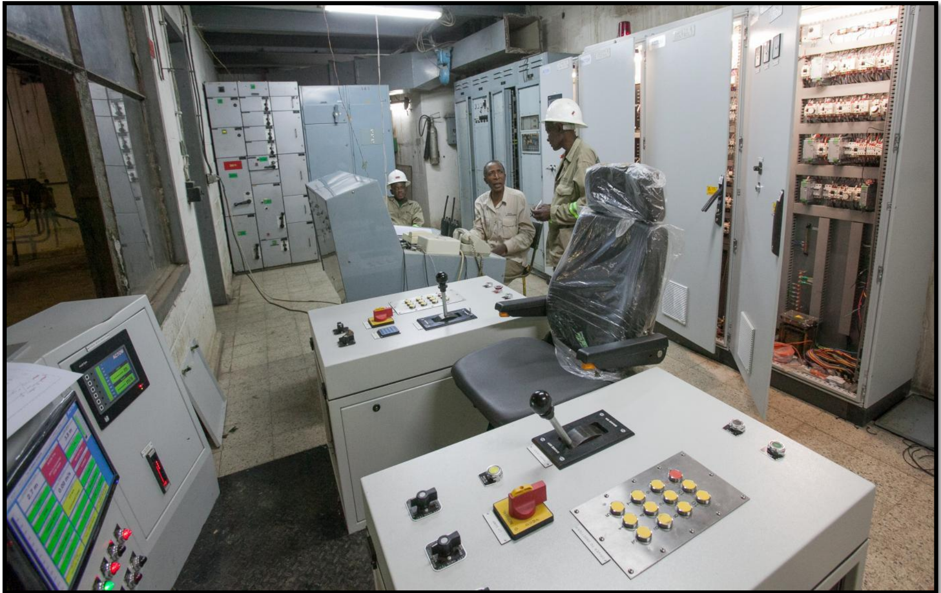
Figure 5: Newly installed winder control centre at Shaft 5.
