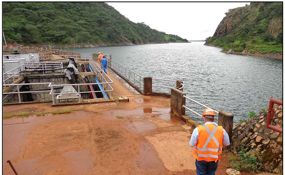
Nzilo 1 hydroelectric power plant, Katanga, DRC
