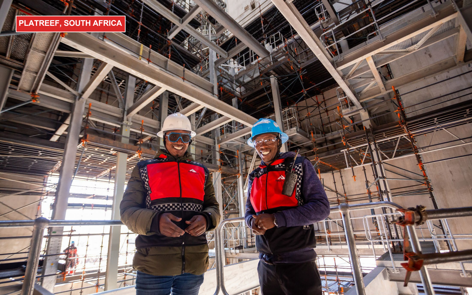
Thomas Shonyoane (left), Risk Officer, and Vincent Mahuangu (right), HSE Officer, members of the Platreef safety team, inspect the interior of Shaft 2 where internal steelwork erection continues.
