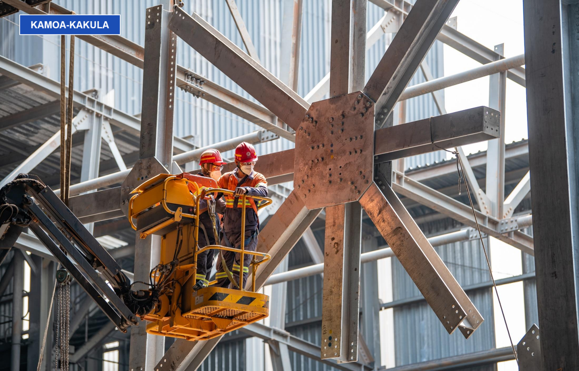
Support structures being installed at the concentrate warehouse for Kamoja-Kakula's fourth Larox filter by contractor KKCC. (L-R) riggers Wai Da Min and Chan Ha.
