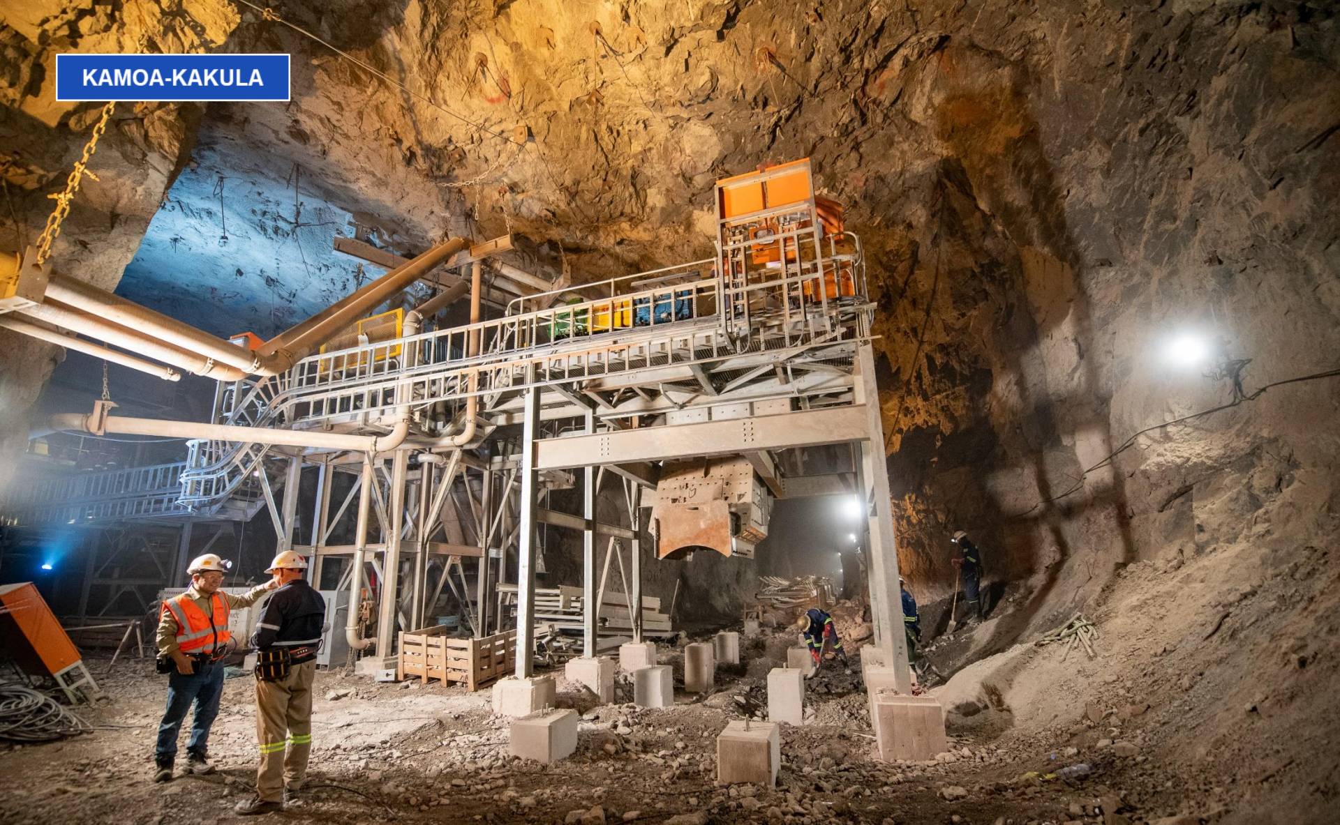
Abraham Li, Director and General Manager (left) explaining construction methodology of the eastern conveyor at Kakula underground.
