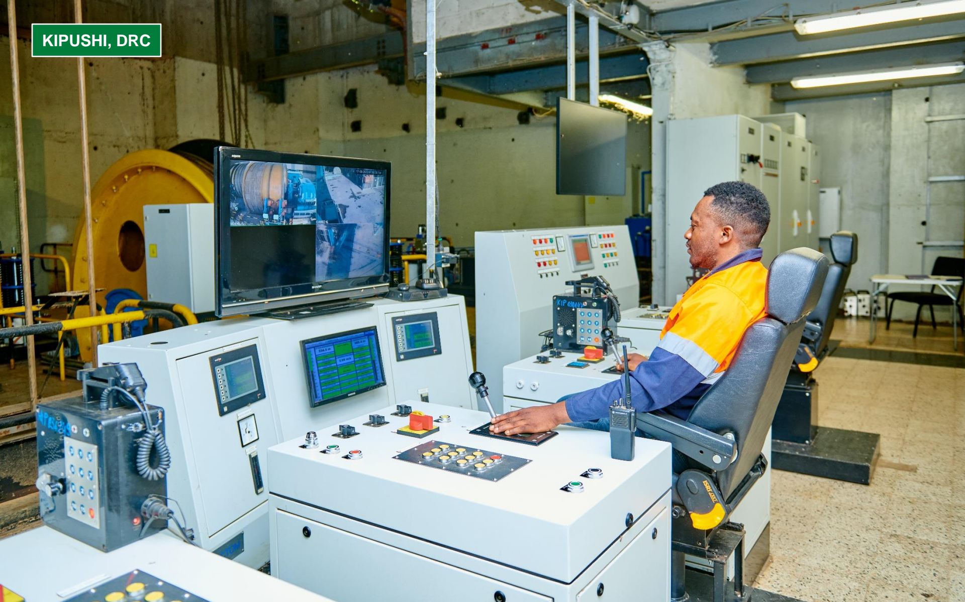
Kipushi employee Bamanya Samuel Bielanshi (winding engine driver), at the winder control desk which transports up to 30 people in the shaft cage from surface to the 1150-level underground.
